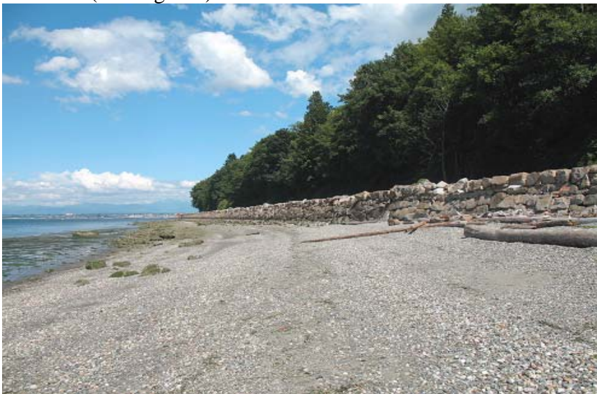
Photo 4: Transition zone between restored and unrestored beach in front of railroad bulkhead (looking east)
